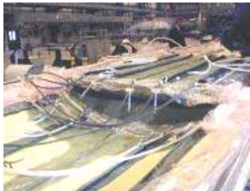
Vacuum infusion of a rail vehicle roof structure (courtesy of Bombardier Transportation)
